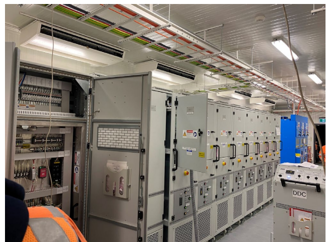
Figure 2 - Energy Storage System installed at Diamond Creek Substation
