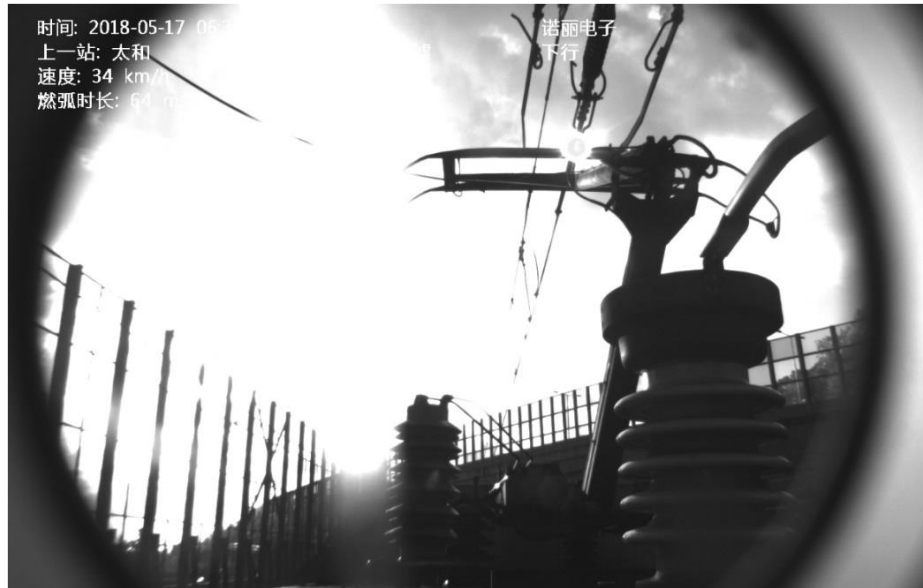
Detect repeated arcing alarms
